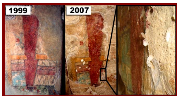
Fig. 1 – Damages caused by the inappropriate application of polymers to Mesoamerican mural paintings.
